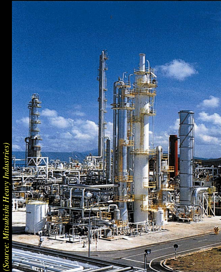
Post-Combustion Capture (gas-fired power plant, Malaysia)
