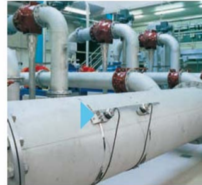
Prosonic Flow (clamp on version shown) is used to control cooling water for the main condenser
